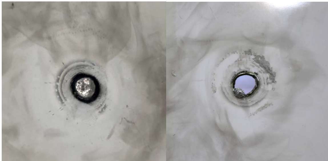
Figure 7: Left: Exterior-side damage, and right: through hole
