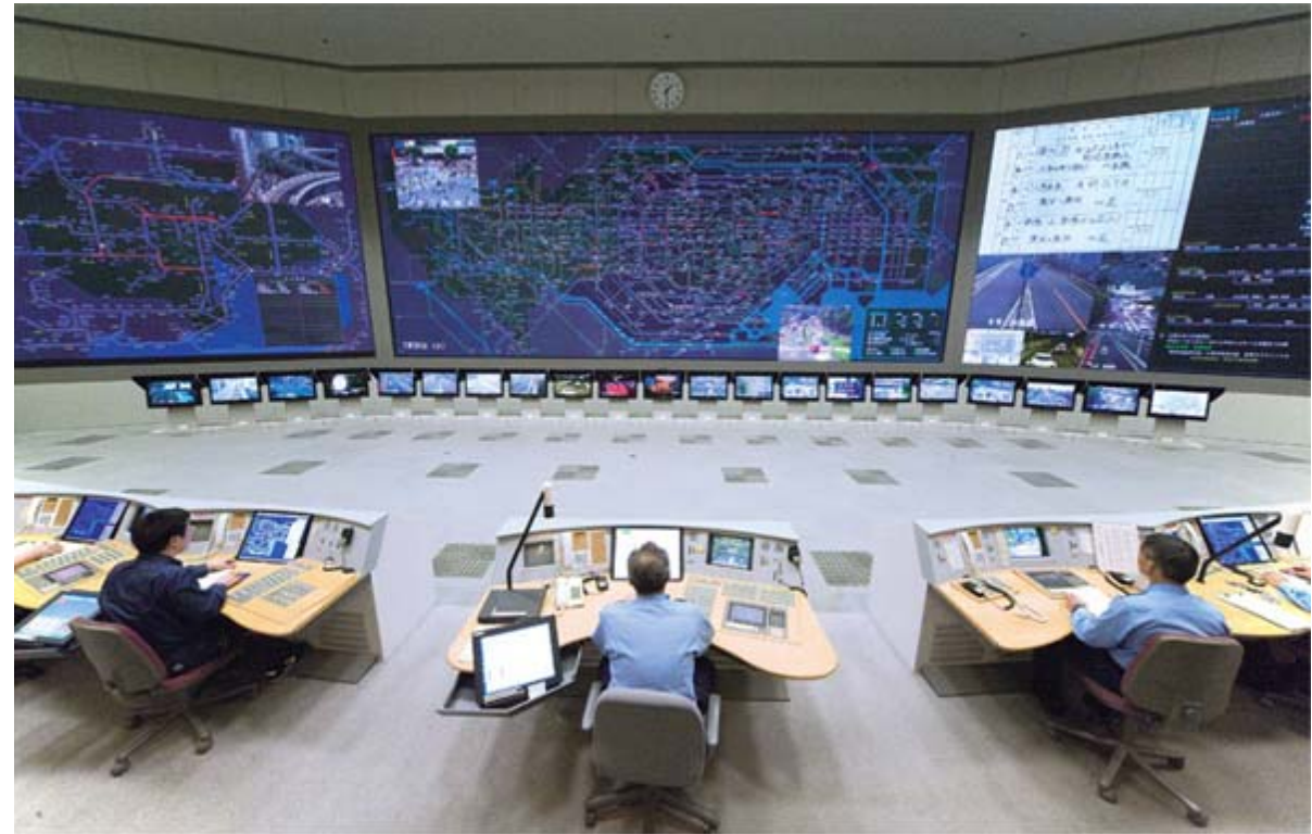
Traffic Control Center
